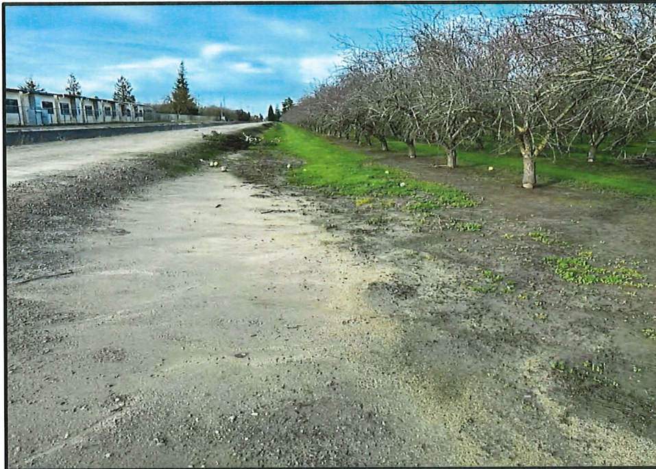
South edge of the site, looking west from the southeast corner of the site; 01/12/23.
